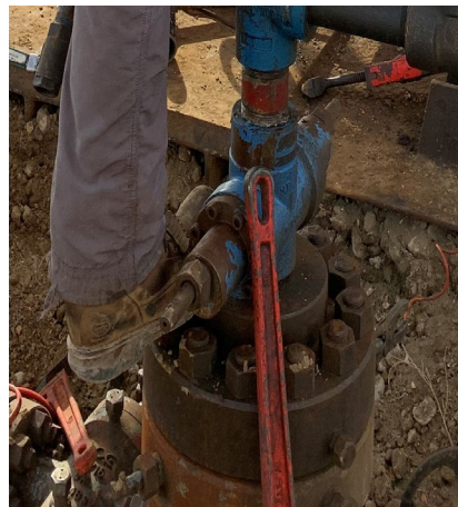
Location of where IP's foot got caught on wellhead.
